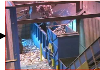
MSW Sorting is made on a mezzanine platform over the Tipping Floor
