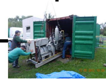
Many Containerized CHP power plants are located within 50km radius of the landfill
